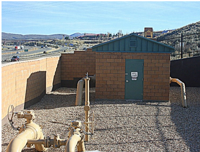
Natural Gas Pressure Regulator Station for 12", 10", 8" inch Pipelines
