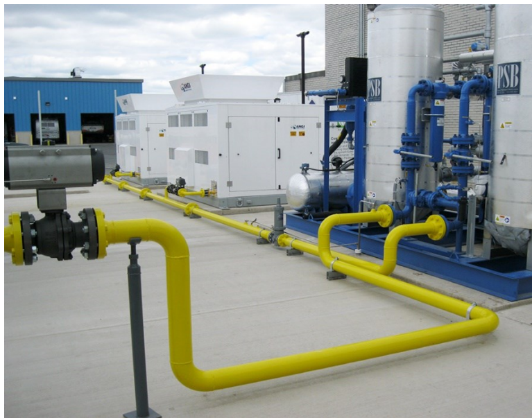
CNG Compressor and Pressure Regulating Units
