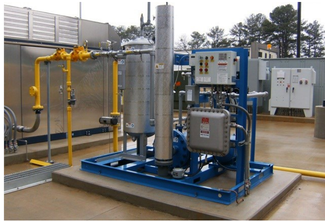
CNG Pressure Regulator @ Fueling Station
