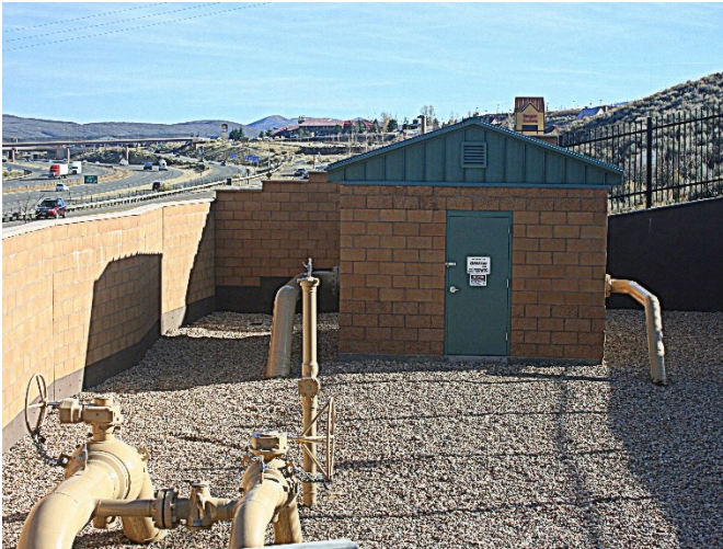
Natural Gas Pressure Regulator Station for 12", 10", 8" inch Pipelines
